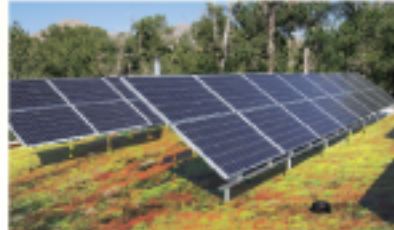
Solar Industrial System
