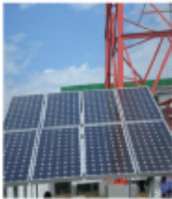
Solar Telecom System
